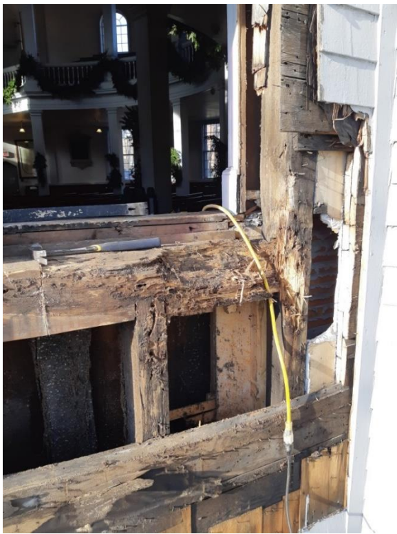
The rotted sub sill
